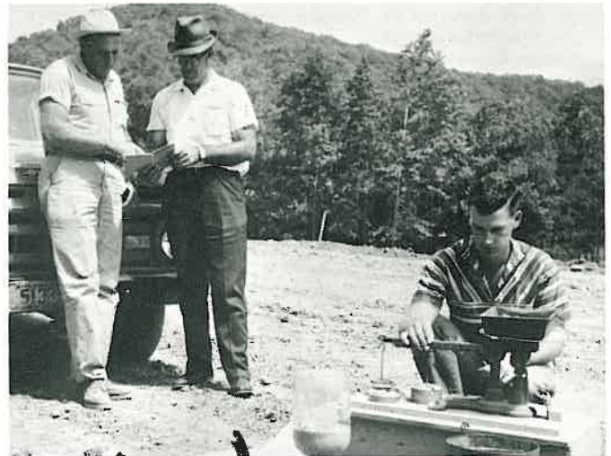
Coleman Stamps, junior inspector; Curtis Pangle, resident engineer; and Frank McCollugh, rodman, are taking a density test east of Highway 16, which is being reconstructed between Pettigrew and Red Star. The men are in District 9.
