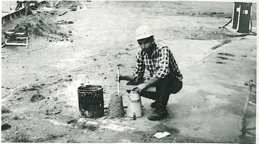
Earl Kirkpatrick, instrumentman in District 2, is shown taking concrete slump tests on Job 2612, Hamburg north reconstruction.
