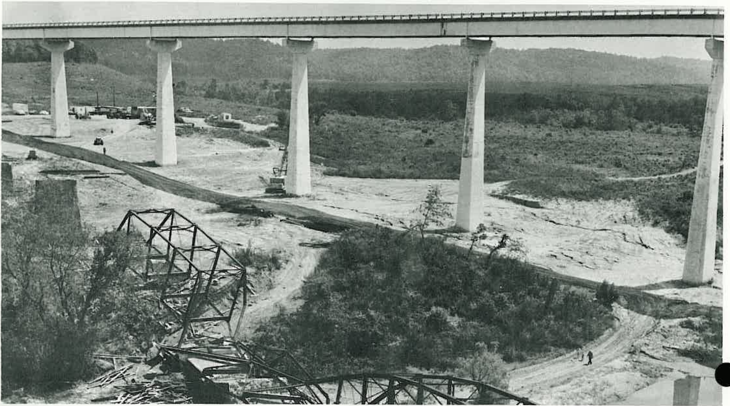
The old bridge in the foreground, completed in 1902, was "blown down" not long ago with the use of 102 sticks of dynamite placed around two of its piers. The new bridge crosses part of Beaver Lake. The scene is looking upstream on the White River on Highway 12, east of Rogers.
