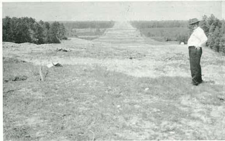
Gayle Gunn, resident engineer in District 7, is shown inspecting the clearing and grubbing which have been completed on Job 7573, Gum Springs, a heavy road section of Interstate 30, south of Arkansas.
